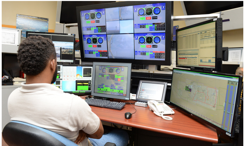
AT THE AIR FORCE'S RIDLEY MISSION CONTROL CENTER, ONE OPERATOR WATCHES UP TO 4 TRACKING SYSTEMS. FEW PEOPLE NEED THIS MANY SCREENS. U.S. AIR FORCE PHOTO BY KENJI THULOWEIT
